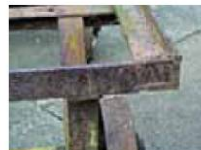
Figure 9.2 A rusting railway trolley (showing pitting)
