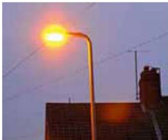
Figure 2.34 Street light (based on sodium vapour lighting)
